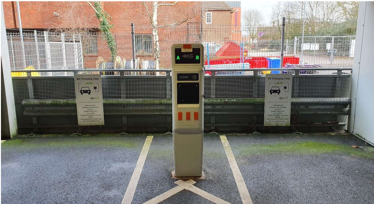
Figure 37 – Example of EV charge point within The Friary Multi-Storey car park
